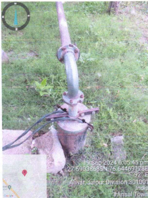
Figure 2 : Photograph of Bore Well 2.
